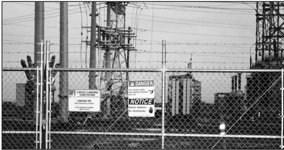
Photo courtesy of Youth United for Community Action. The Cooley Landing Substation site is shown behind a locked fence on Bay Road near Cooley Landing in East Palo Alto.
