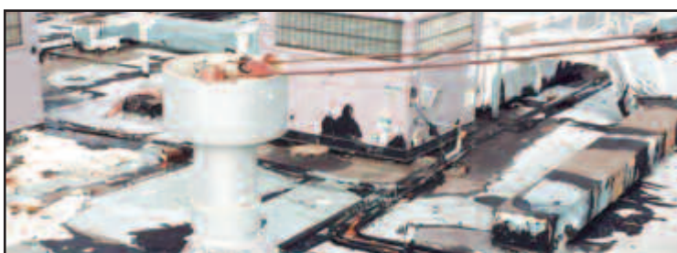
Photo by Ravenswood City School District This photo shows some of the roof repairs that are needed.
