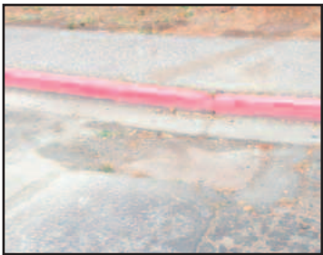
Photo by Ravenswood City School District Pothole needing repairs
