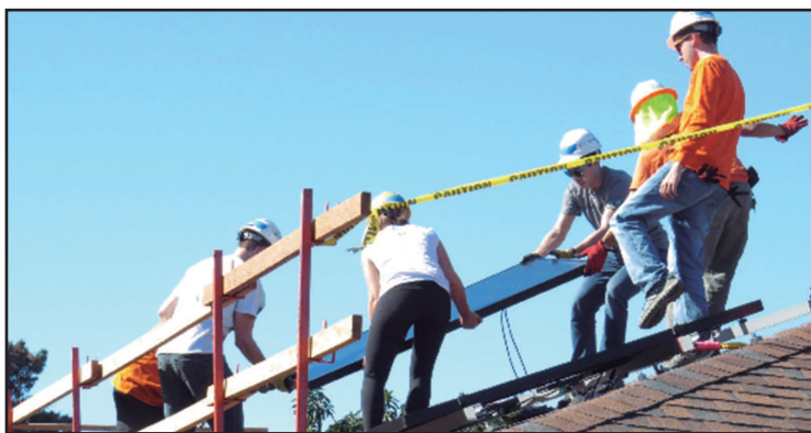
This team shows how the panels are brought up to the roof and positioned for installation.
