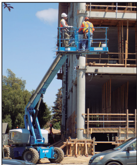
Workers prepare to attach portions of the pre-cast brick exterior to the sides of the building.
