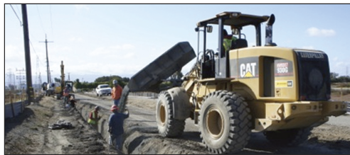
Photo courtesy of Peter Geraghty Construction is shown taking place along the access road to Cooley Landing Park
