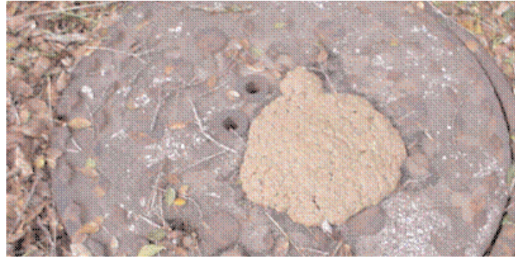
A manhole oozes grease from a blocked sewer line. Pictures courtesy of Regional Water Quality Control Plant.
