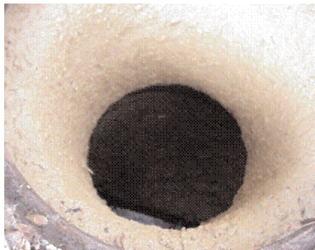
A peek underneath a manhole cover shows grease and oil build-up inside a sewer line.
